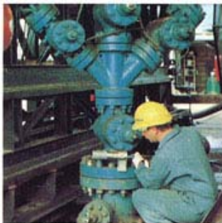
Tightening bolts on Christmas Tree.
